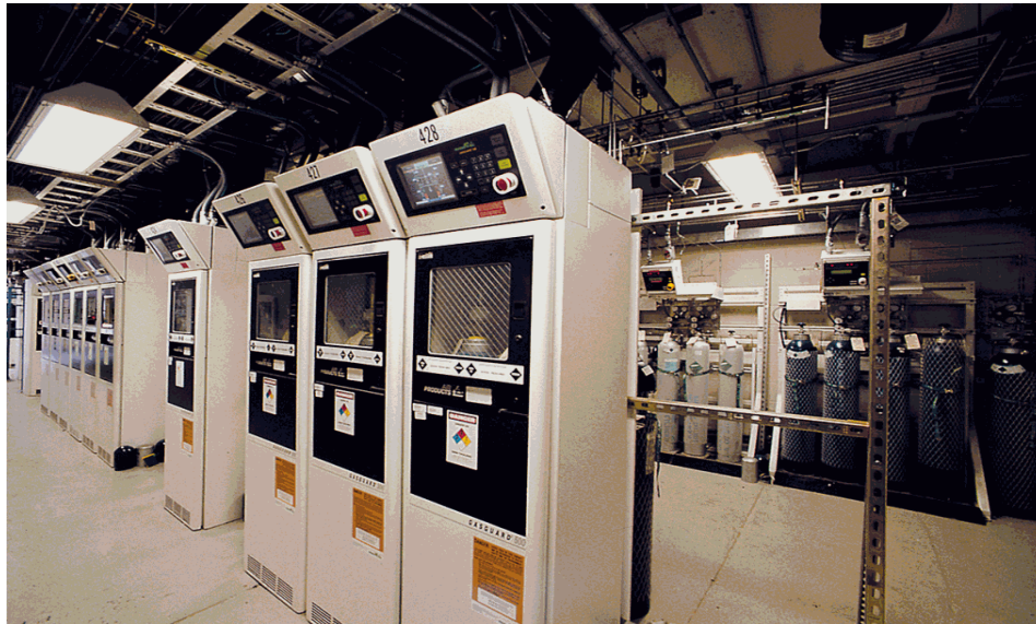
Figure 1. GASGUARD System at a Semiconductor Facility
